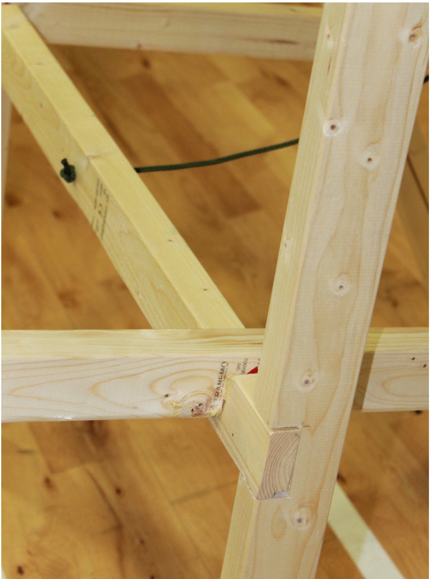
Detail of front cross bar, front leg (half-lap joint), and support arm. The support arm is not quite fully in place, hence a small amount of the "tell tale" red paint is still visible.
